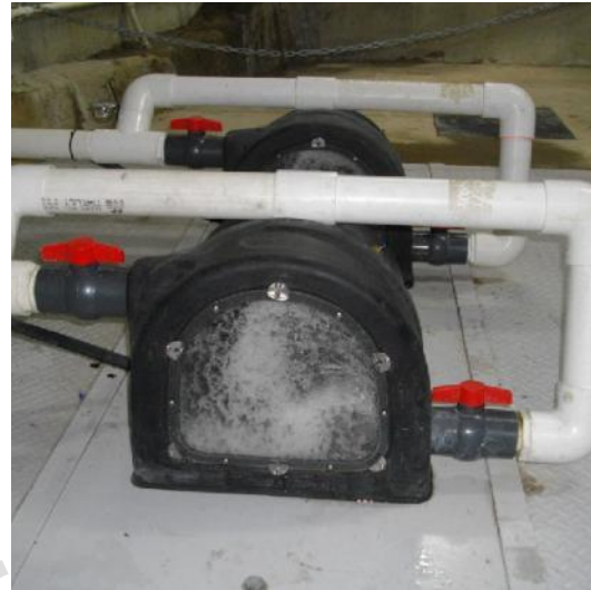
Typical good commercial install – power for reservoir Auckland city storage
