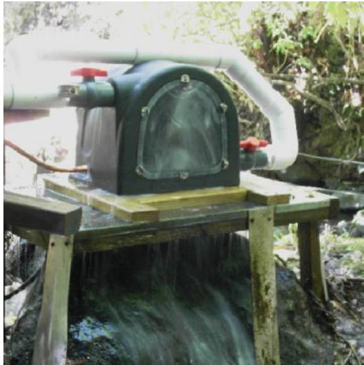
Typical good domestic install on natural rock foundation
