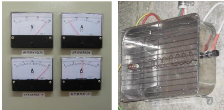
Standard meter cabinet and resistive load
