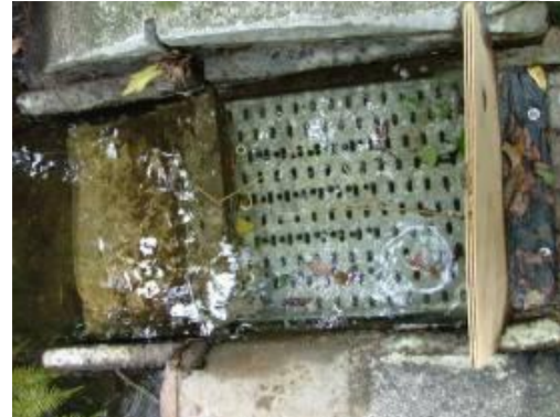
Perforated galvanized cable tray intake
