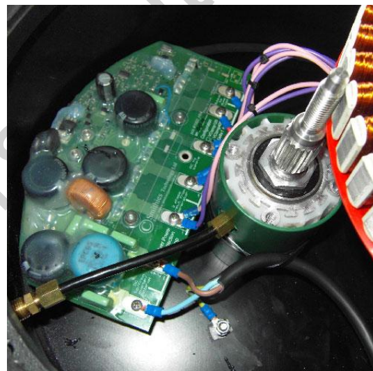
Delta connection from a 6-Wire generator ME or GE PowerSpout
